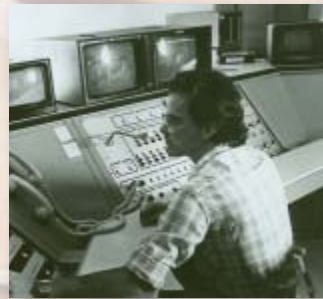
State-of-the-art in 1981: the Inter Terminal Train Control Room.
